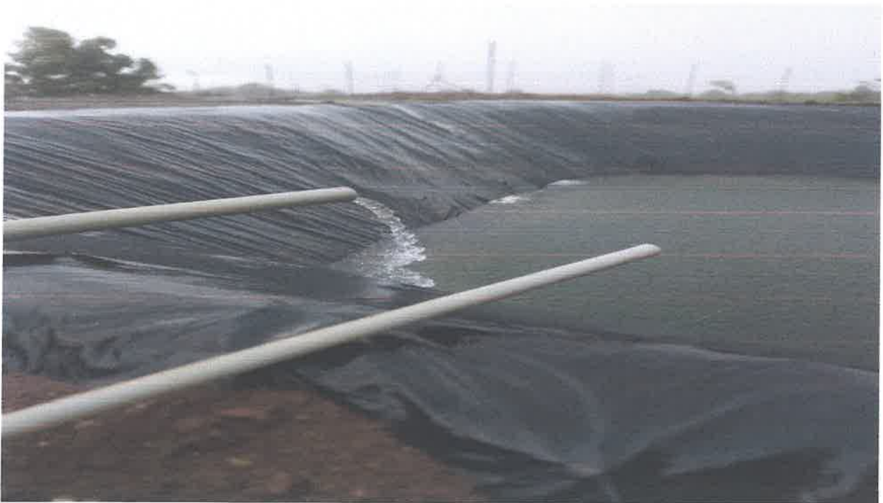
Filling water in the farm pond with roof water harvesting during monsoon
