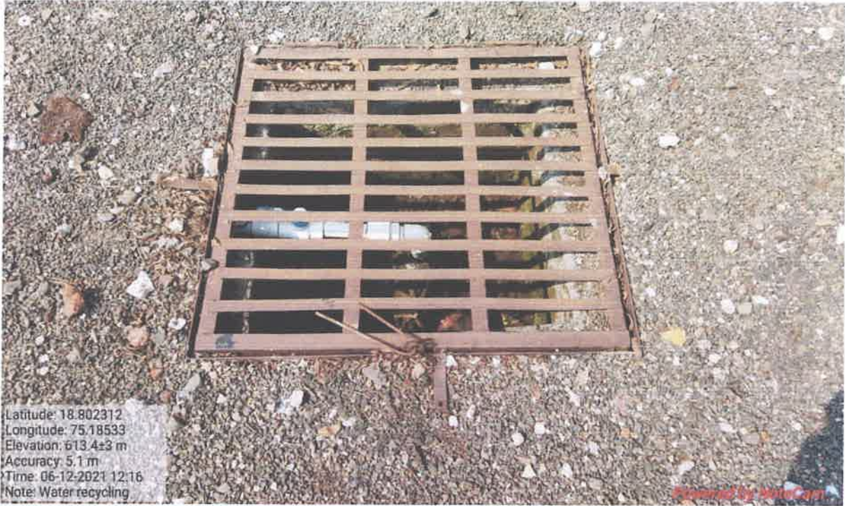
Roof Water Harvesting
