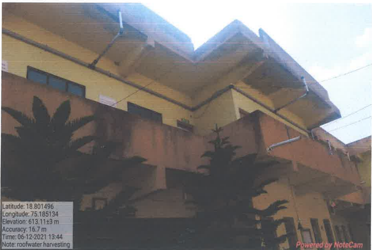
Rain Water Harvesting
